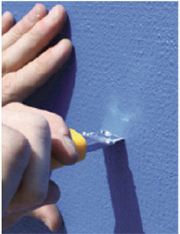
Using a sharp blade, cut a 30mm slot, 50mm deep into the wall.
